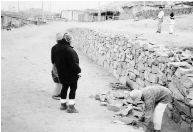
Residents constructing stabilization walls in one of the shanty towns outside of Lima, Peru.
